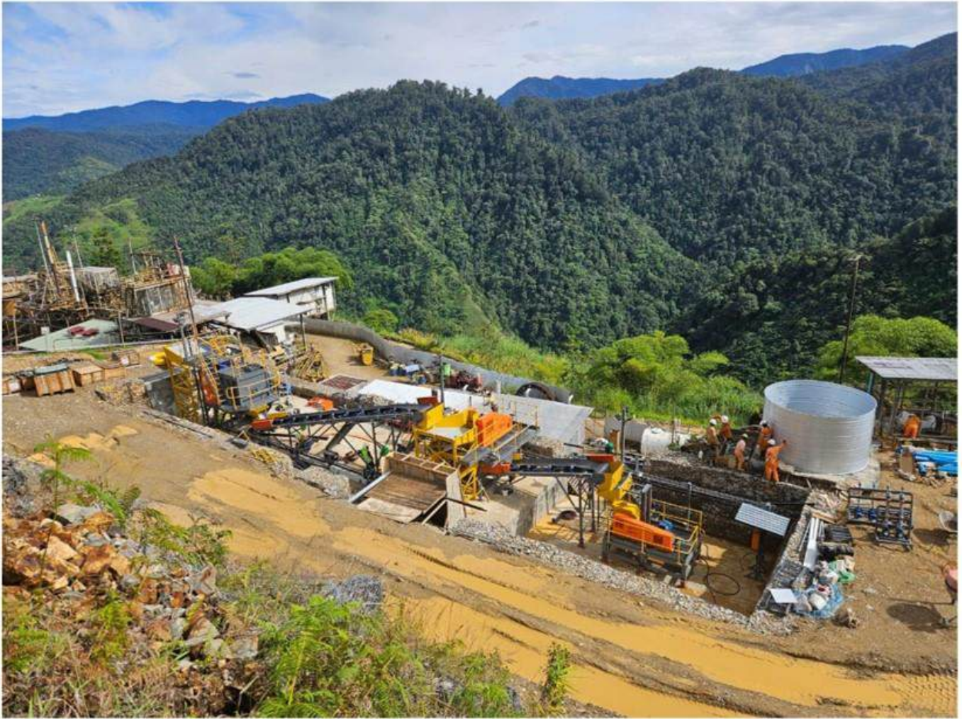
Figure 26 - Modular gravity plant installed, photo taken December 2024
