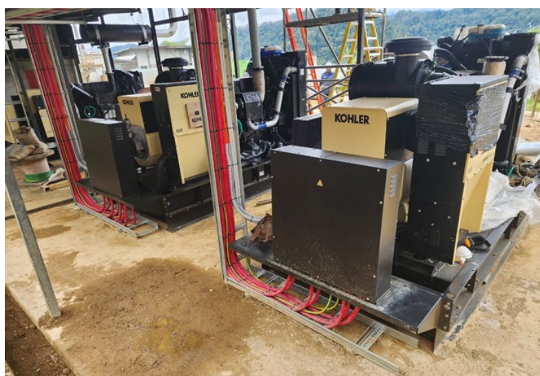
Figure 4: 1.3 MW power station at Tolukuma
