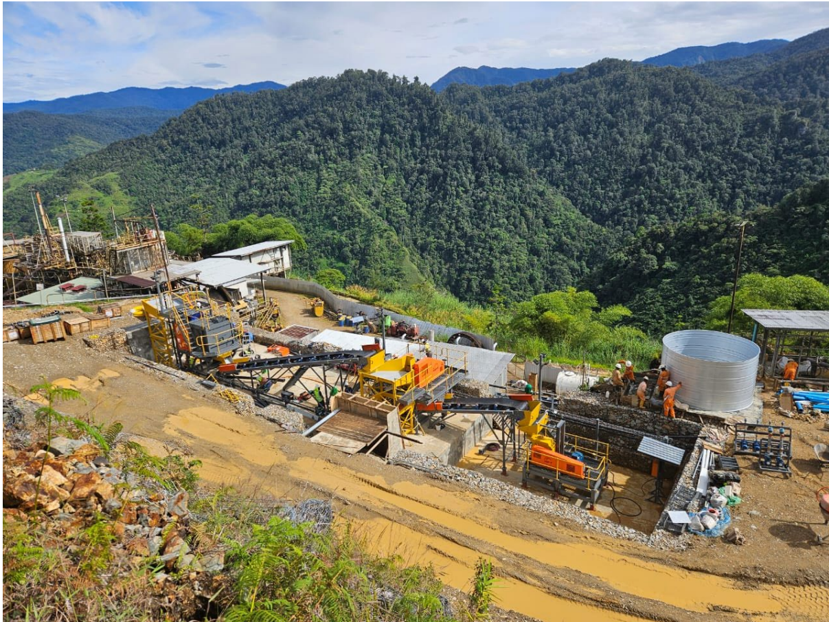
Figure 2: APT modular plant Installed, December 2024
